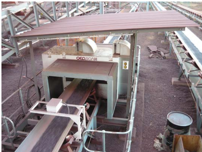
Figure 1. Elemental analyser and moisture monitor installed in an iron ore processing plant.
